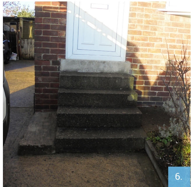
Unsafe exterior steps with no guarding.
