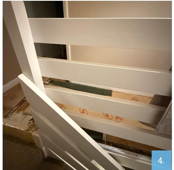
Horizontal balustrading spindles, easy to climb.
