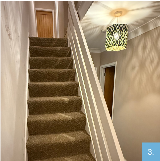
Climbable horizontal balustrading, needs a handrail on the left.
