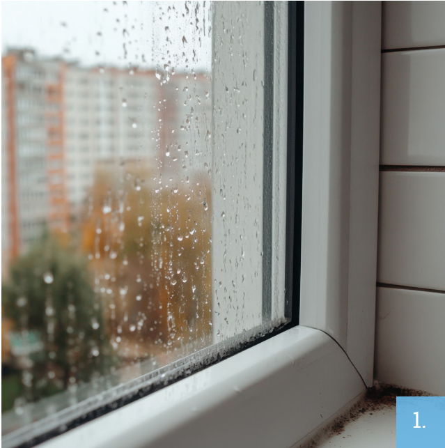
Condensation on a window with mould forming on the windowsill
